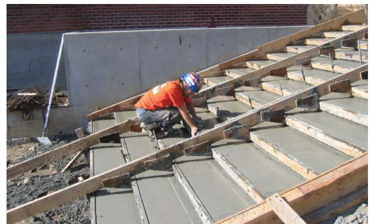
June 2007: Concrete for the grand stair is poured at the east entry.
