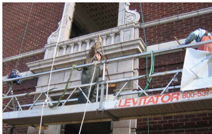
June 2006: Terra cotta and brick on the historic structure are cleaned and repaired.
